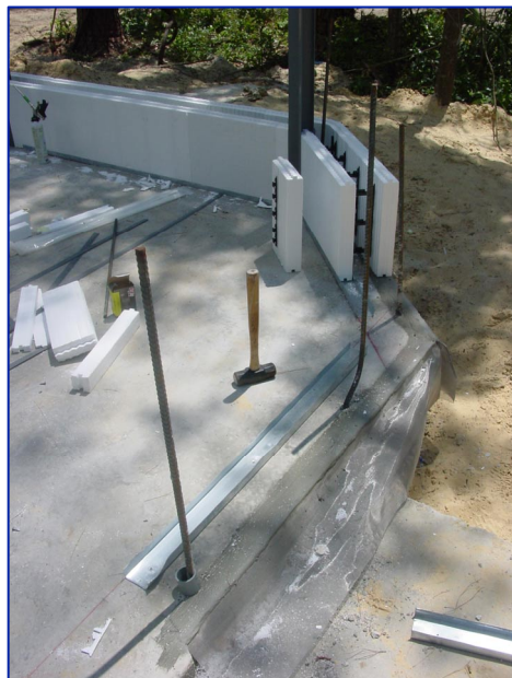
ECO-Block ICF wall being installed in the Madera Model embedded rebar and Termimesh subsurface poison-free termite barrier visible.
